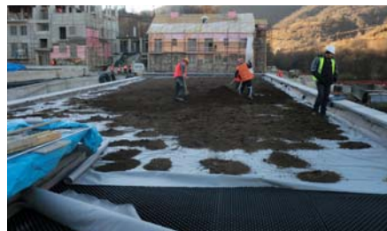
The substrate which was mixed on-site previously was applied all over the system filter.
